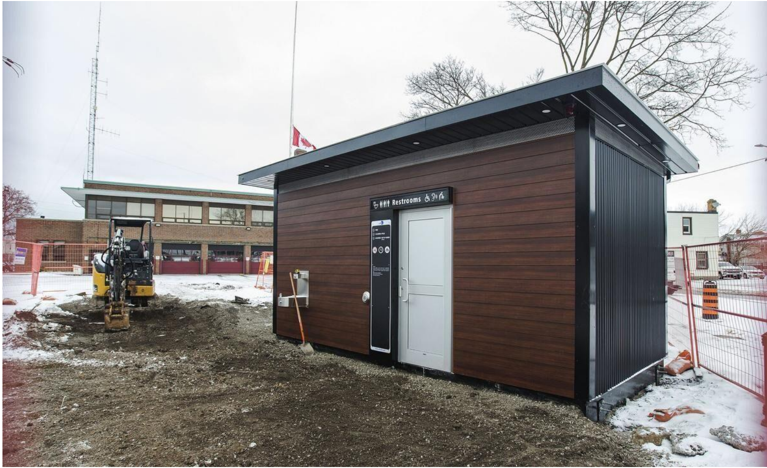
A self-contained public restroom is being installed at the intersection of St. Paul, Geneva and Niagara Streets. Bob Tymczyszyn / Torstar
