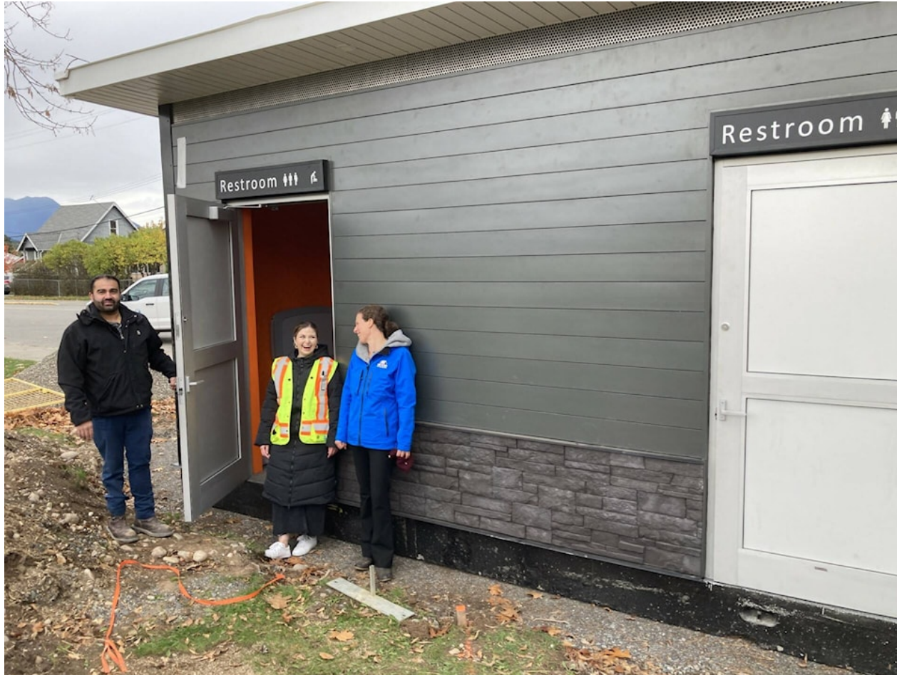
That's City of Terrace parks and recreation facilities manager Monty Gill on the left at the new washroom building being installed at George Little Park. In the middle is Reanna Fyley from building provider Parkworks and on the right is Tara Irwin, the city's parks, recreation and culture director. (Staff photo)
