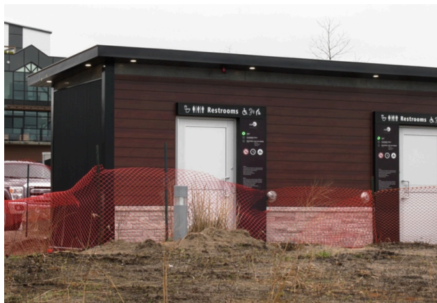
New smart washroom facility being installed in Grand Bend. April 17, 2024. (Bryan News London)
