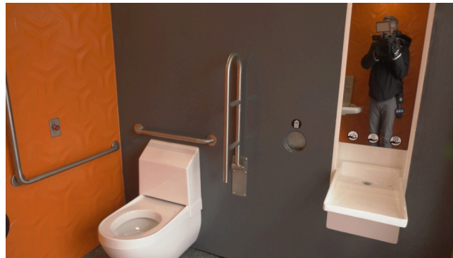
New smart washroom facility being installed in Grand Bend. April 17, 2024. (Bryan Bicknell/CTV News London)
